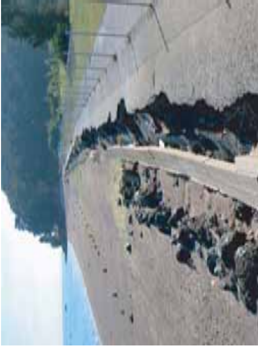
A - Collapsed promenade curb
